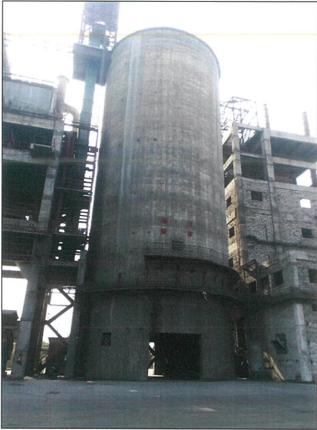
LINE 3 Cement Silo
